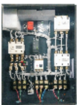
Interior View of MU-G30W FASD
