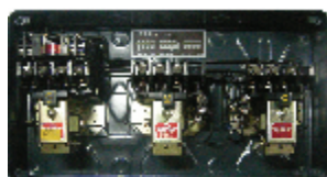
Interior View of MK1 SASD
