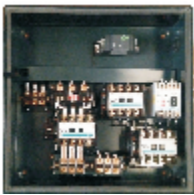
Interior View of MU-G20W FASD
